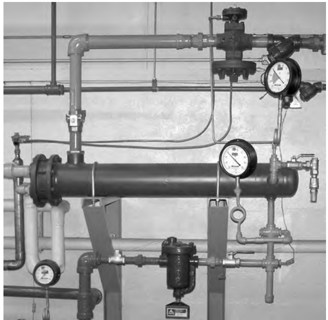
Feedback instantaneous systems suffer from lag time, tube bundle corrosion and problems with thermostatic element deterioration.
