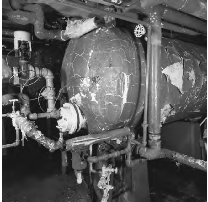
High-maintenance feedback systems with bulky tank units like this one often leak, corrode or rupture a thermostatic control.
